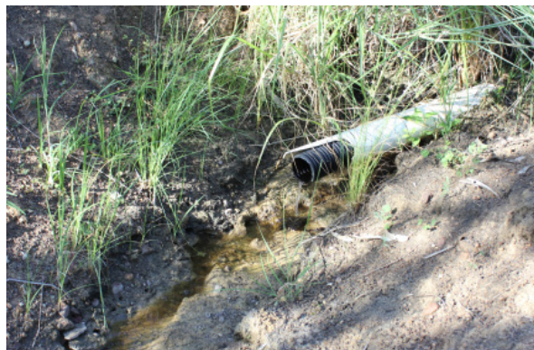
Pictured: Layton Mitchell has layered river sand and perforated pipes in trenches to divert excess surface water from low lying areas. He has a small herd of cattle on the farm's higher, grassy slopes.
